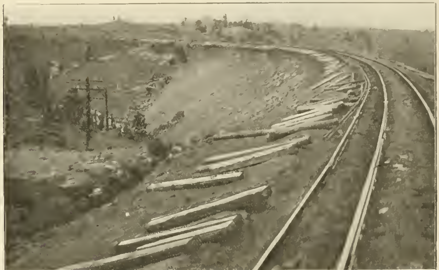
"LONE TREE" FILL. UNION PACIFIC. 400 FT. WIDE AT BOTTOM, 8 FT. WIDE AT TOP.
